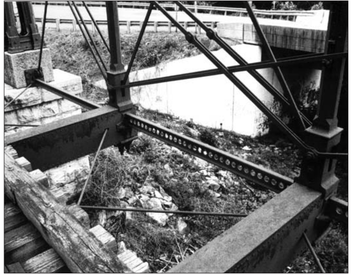
A portion of the lower chord, floor beams, and cross bracing. (Michael Caplinger, 1999)
